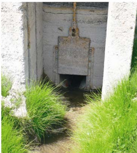
Photo 4: Concreting of the bottom boards of the monk at Ribières Pond with a pipe through it (photo L. Touchart, 2006)
