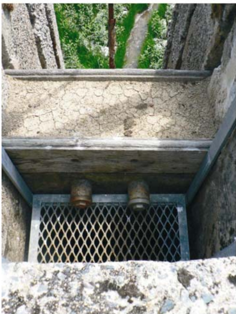
Photo 3: Space between two internal rows of boards in the monk at Ribières Pond filled with clay (photo L. Touchart, 2006)
